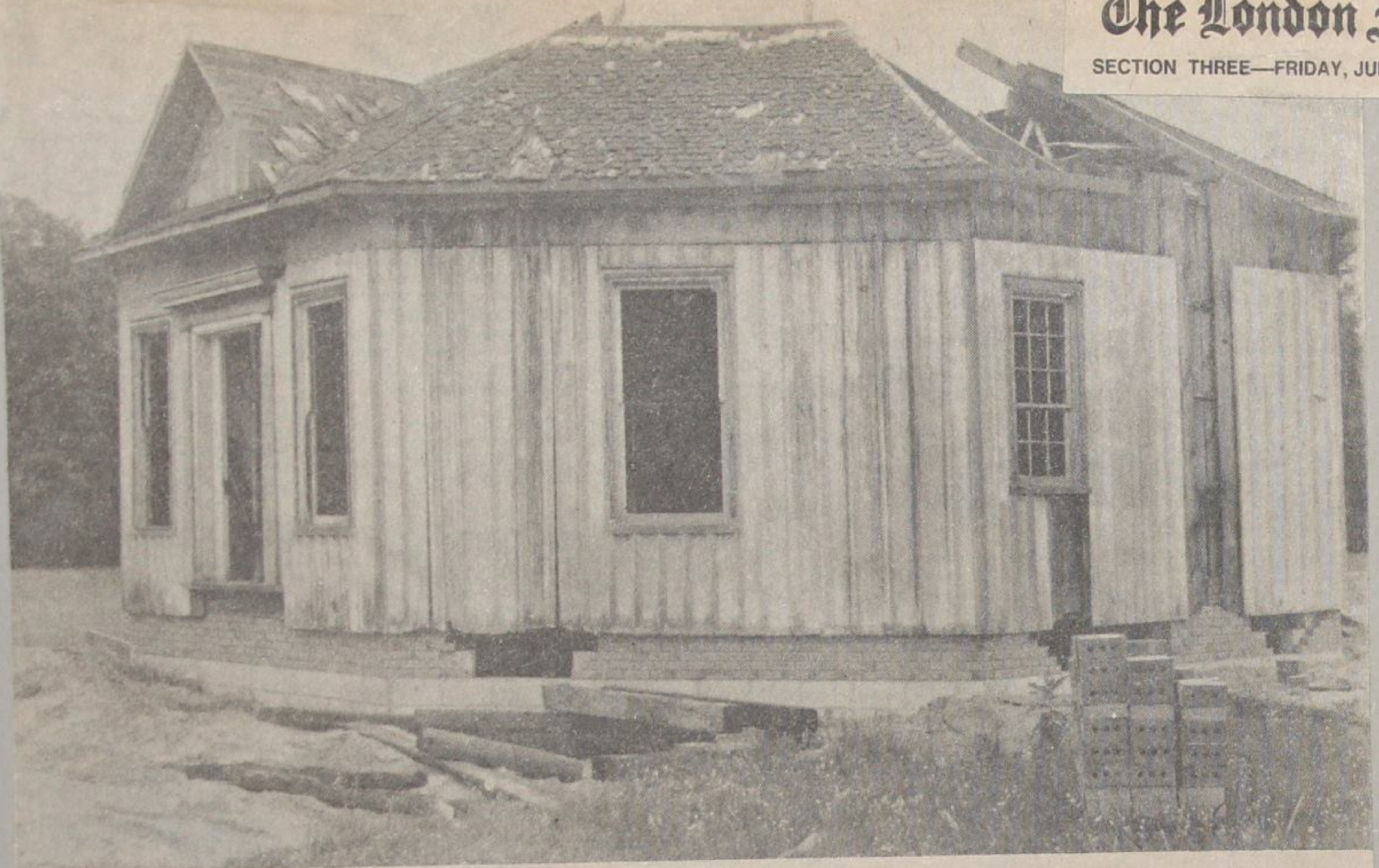
This dilapidated 116-year-old cottage near Otterville may soon become a new meeting place for area senior citizens, if a $40,000 renovation project launched by Norwich South Heritage Committee succeeds. (Photo by Williams)
