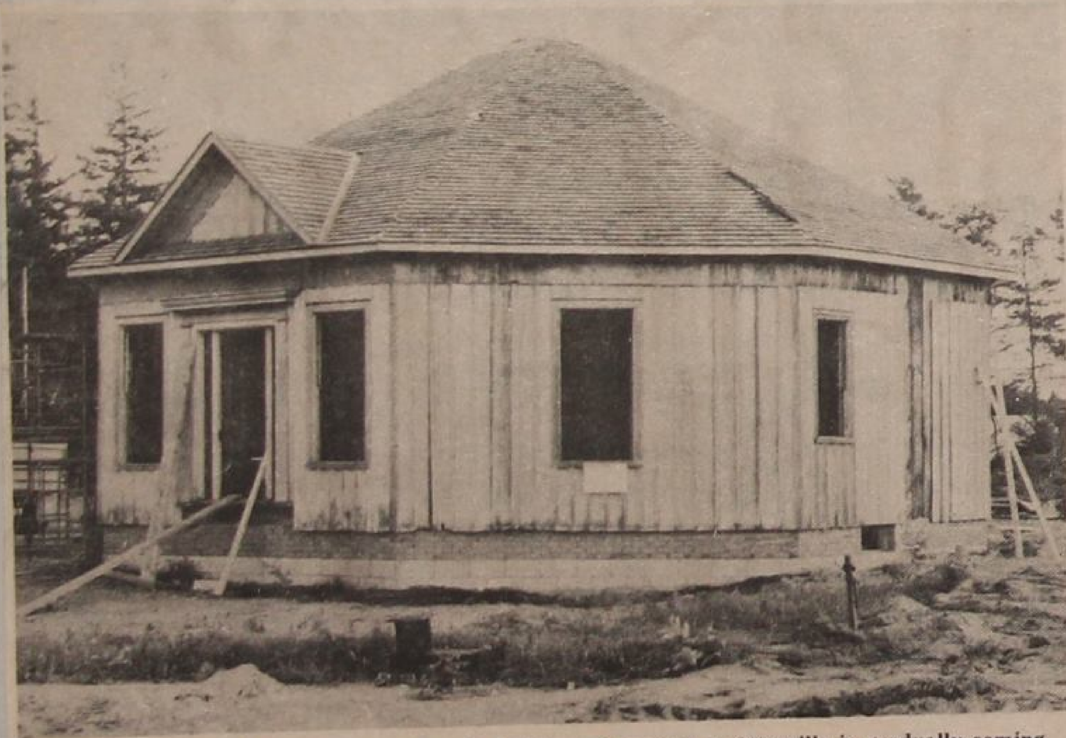
Sporting a new roof the Oddy House at the Erbtown Cemetery in Otterville is gradually coming together. Rebuilding the old hexagonal house is a project of citizens groups in Otterville.
