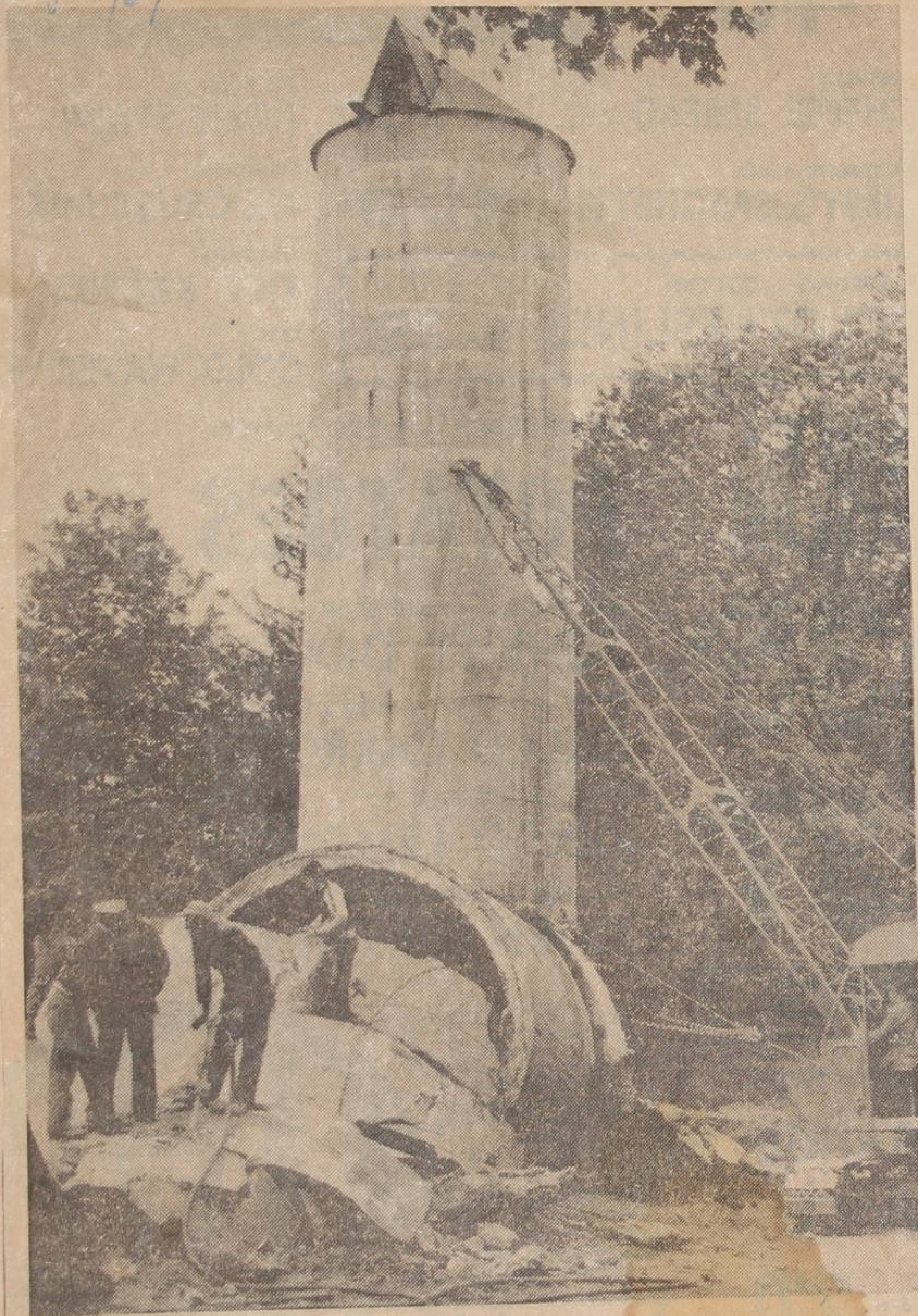
Two old Otterville water towers have fallen to workmen's hammers to make room for a parking lot behind the community centre. Here crews break up slabs in the first before going to work on the second. (Photo by Lowe.)
