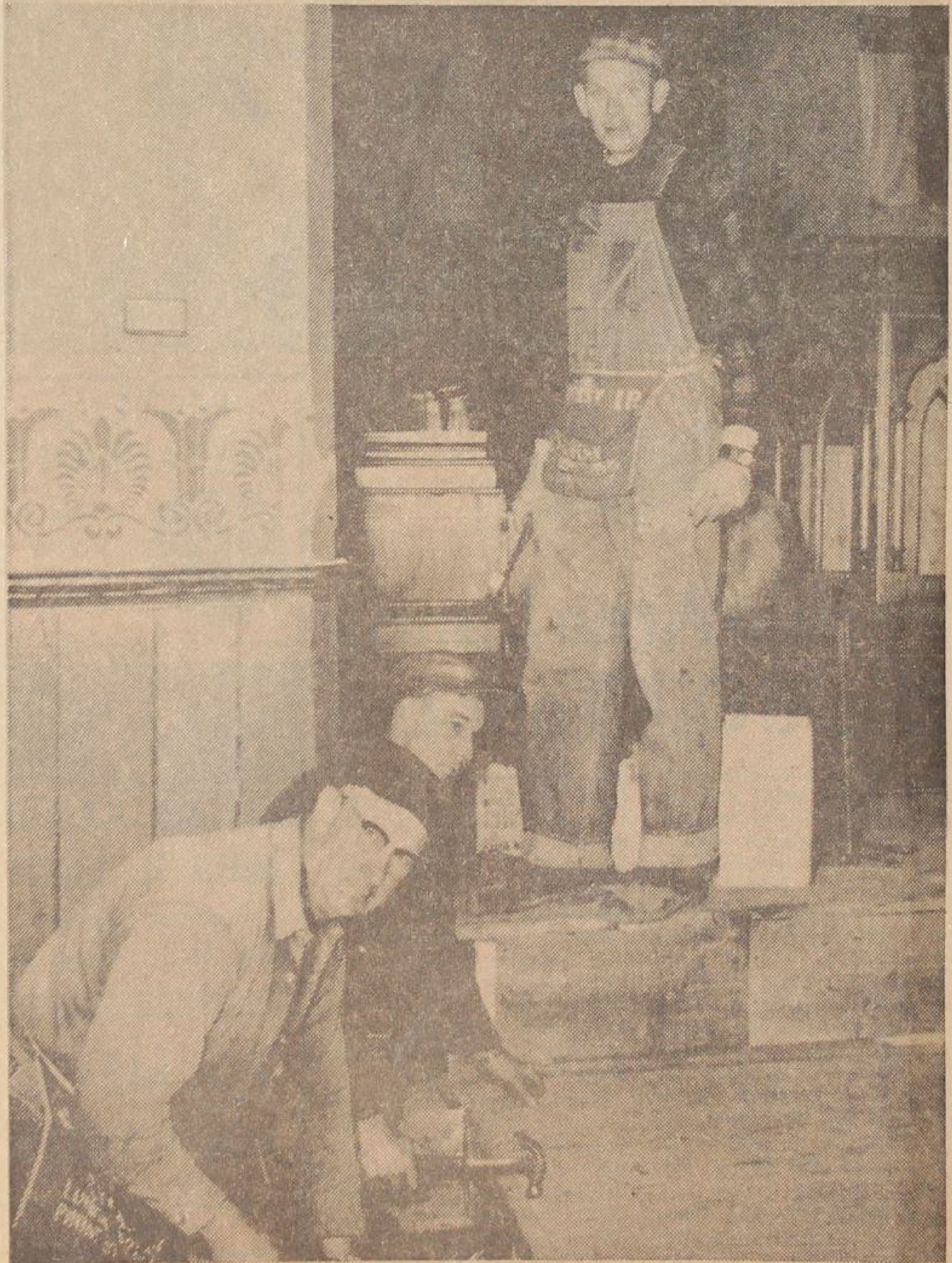
An expected "shoring" task at Holy Trinity Church, Norwich, developed into a major renovation job and many members of the congregation are assisting the work on a voluntary basis. Here, from left, Joe Graves, Fred Slosse and George Duma take part in repairing the church's deteriorating interior.
