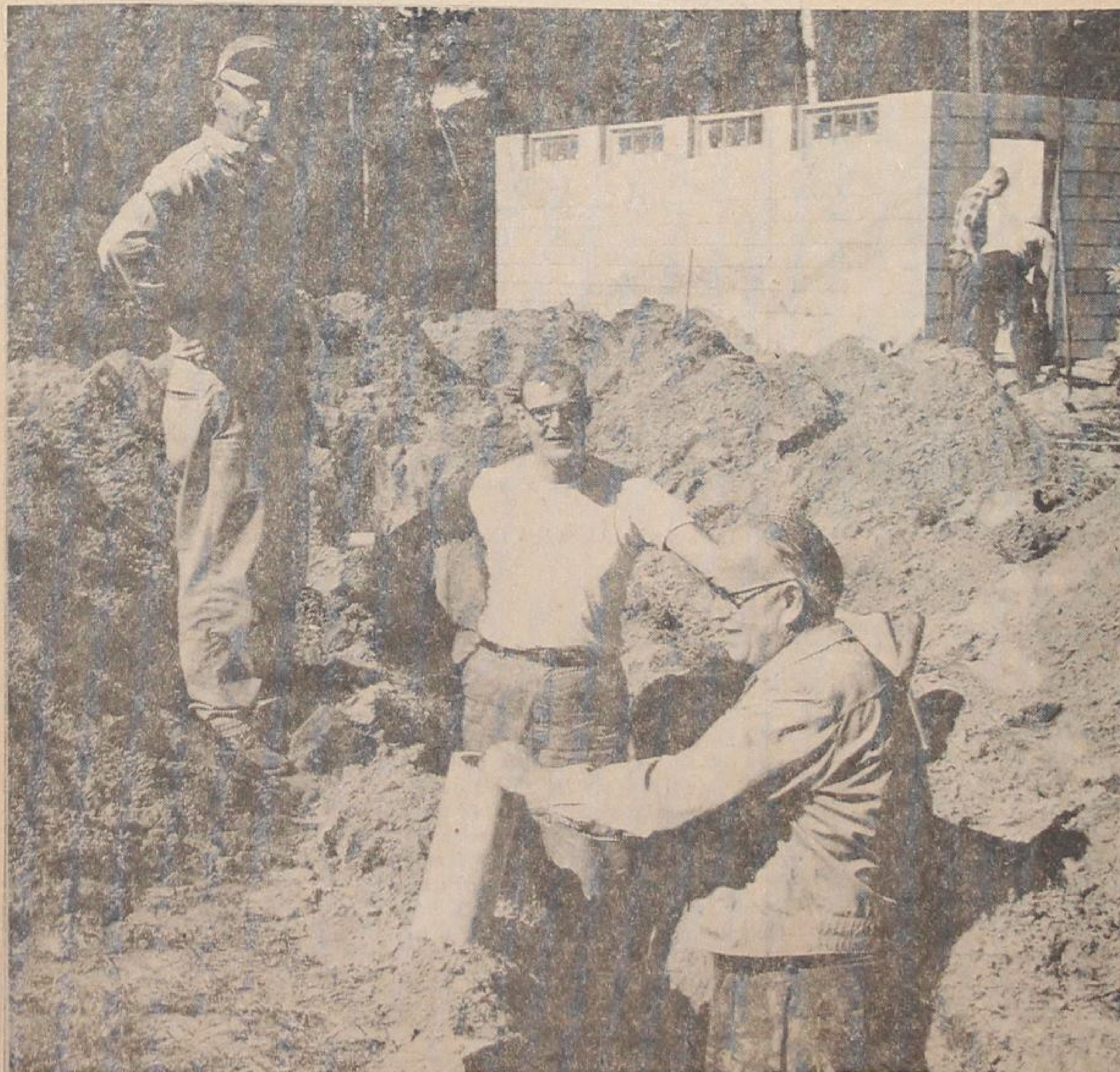
A new public restroom at Otterville Community park is this year's major project for the Otterville-Norwich Lions Club. Cost of materials for the new facilities is
