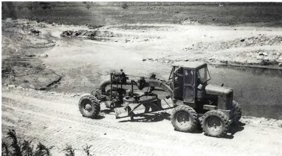
Building the dike, 1949, to re-route the Thames River between Beachville and Ingersoll.
