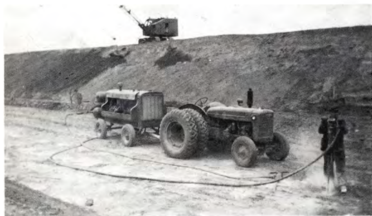
New man-made dike, 1949. In the Spring of 1950 the heavy flow of water tore its way through the new dike back into the old river channel. Repaired.
