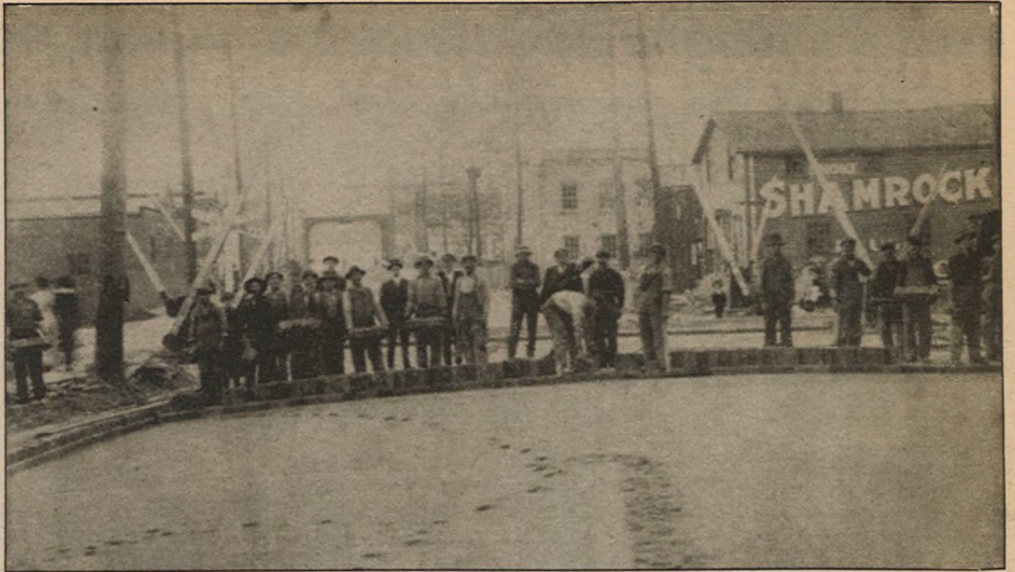
These men are preparing to put down Ingersoll's new road --- a brick one. This photo was taken in the early 1900s.
