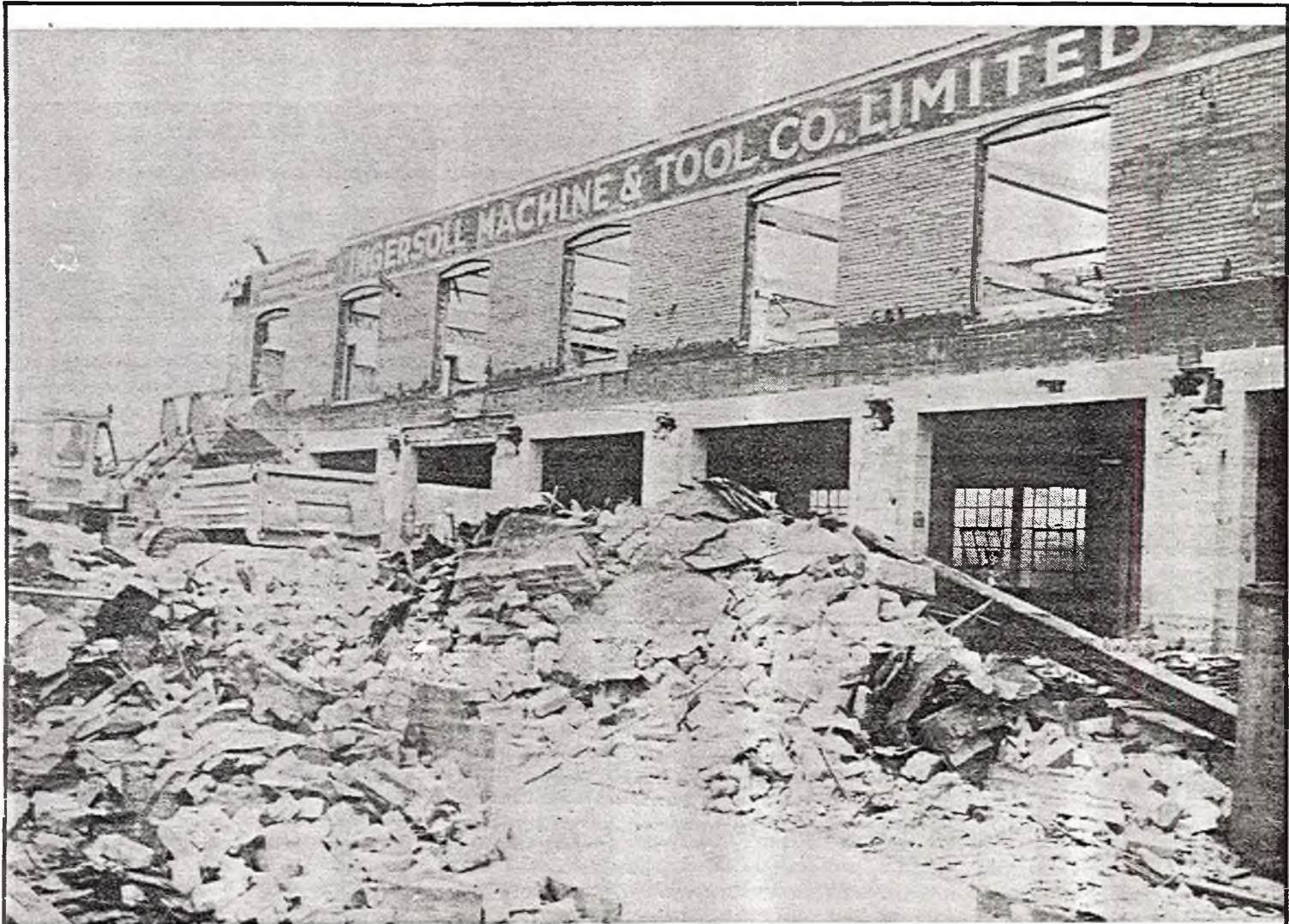
The old Ingersoll Machine and Tool building on King Street West will no longer be standing at the end of the week. It was there in 1912 when the local machine company arrived. It is expected to
