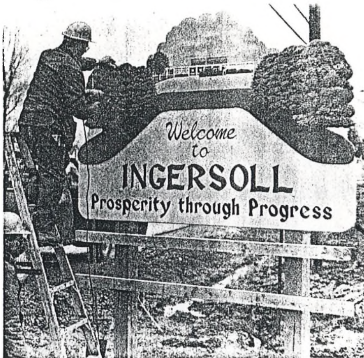
PUBLIC WORKS employee Gerald George installs one of six new welcome signs at the King Street West entrance to town.
