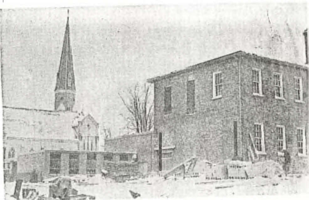
Major changes are under way at the intersection of John and Bell Streets, with a $140,000 wing, above, rising at Sacred Heart Separate School. Opposite the school the new $72,000 Henderson parish hall is almost complete.
