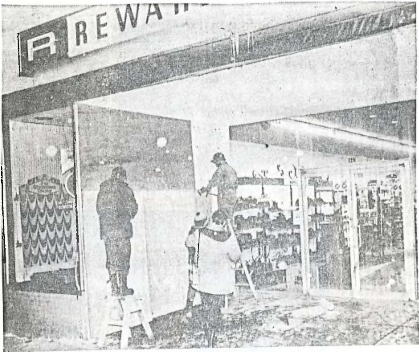
WORKMEN BOARD up window of downtown store after glass - shattering blast last
