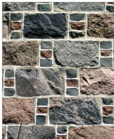
FIG. 16. CRELLIN'S ABERDEEN BOND STYLE MASONRY, WITH 3 SNECKS, MCCORQUODALE HOUSE, 1 29 TH LINE, NO. 6565, NEAR HARRINGTON, OXFORD COUNTY. | KAREN E. ARMSTRONG.
