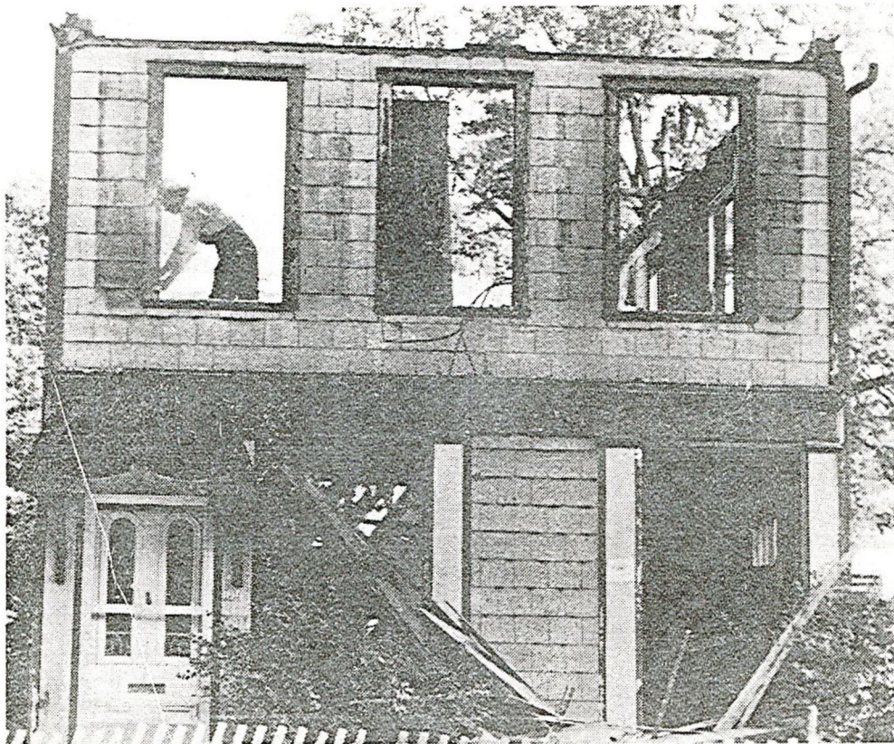
Mennonite farmers worked throughout the week tearing down this century-old house adjacent to the Trinity United Church. The church now has room to expand its parking facilities, while members of the Mennonite community have wooden planks that will be put to use in their homes.
