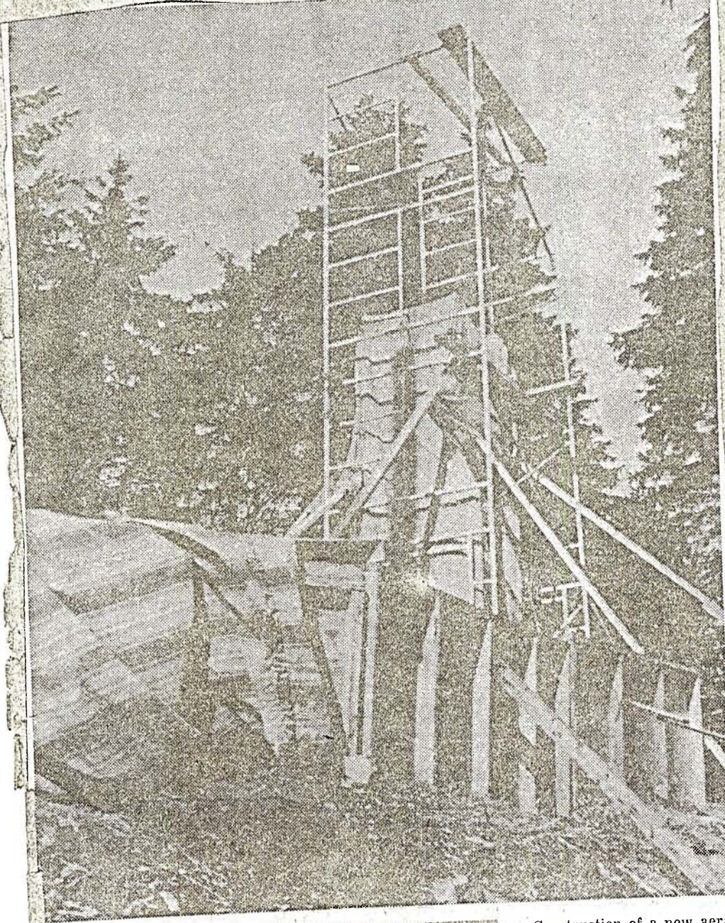
Construction of a new aerator, on Merritt Street, which cleanses the sulphur gas from the town's water supply, got underway yesterday. The project is the first step towards the new $381,000 town water works system. The old aerator is located at the top of the old standpipe in the background. Previous 1970
