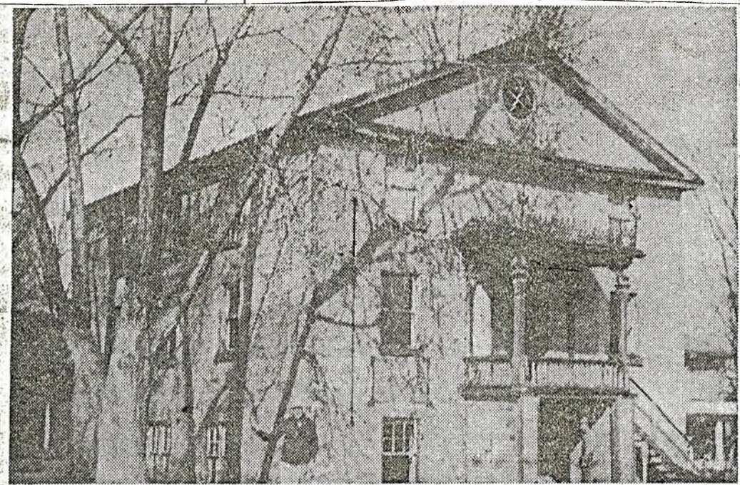
This is the old Wesleyan Methodist Church on Ingersoll's Oxford street, now in the hands of wreckers. The church was once the most northerly terminus of the "underground railroad" for Negroes escaping slavery in the United States. (Photo by Stanley Smith).
