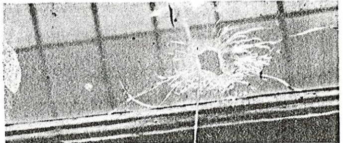
PICTURE SHOWS where bullet went through the window at the Ingersoll police building.
